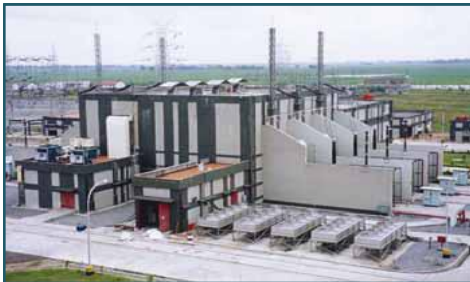
Figure (2.18): 500MW Back-To-Back HVDC System Converter Station [23]
