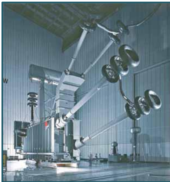
Figure (2.20): A HVDC Converter transformer [24]
