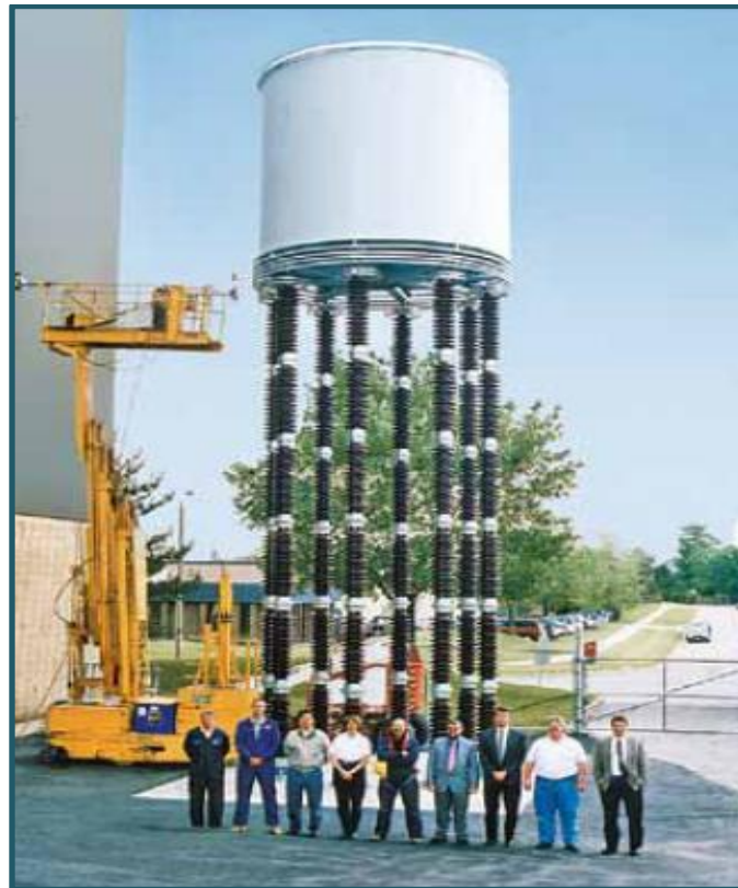
Figure (2.22): Air-insulated dc smoothing reactor, Inductance: 150 mH, Rated voltage: 500 kV DC, Rated current: 1800 A DC [24]
